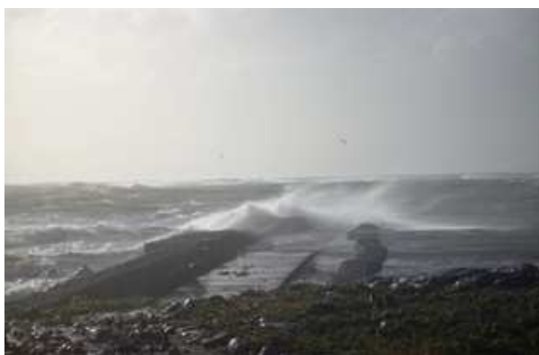
High seas damaged the jetty at Bird Island
